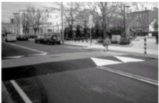
A raised pedestrian crossing provides a continuous route for the pedestrian at the same level as the sidewalk. Pavement markings on the slope (inlay
